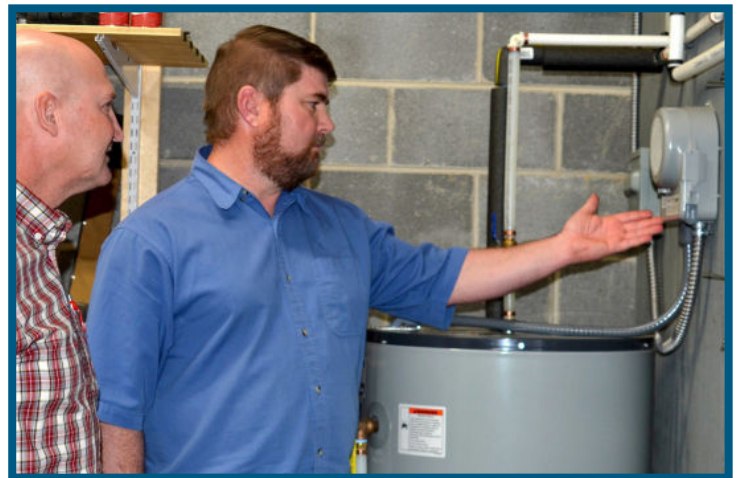
Pictured: A BrightRidge technician explains the TALO device installation on the customer's water heater.
